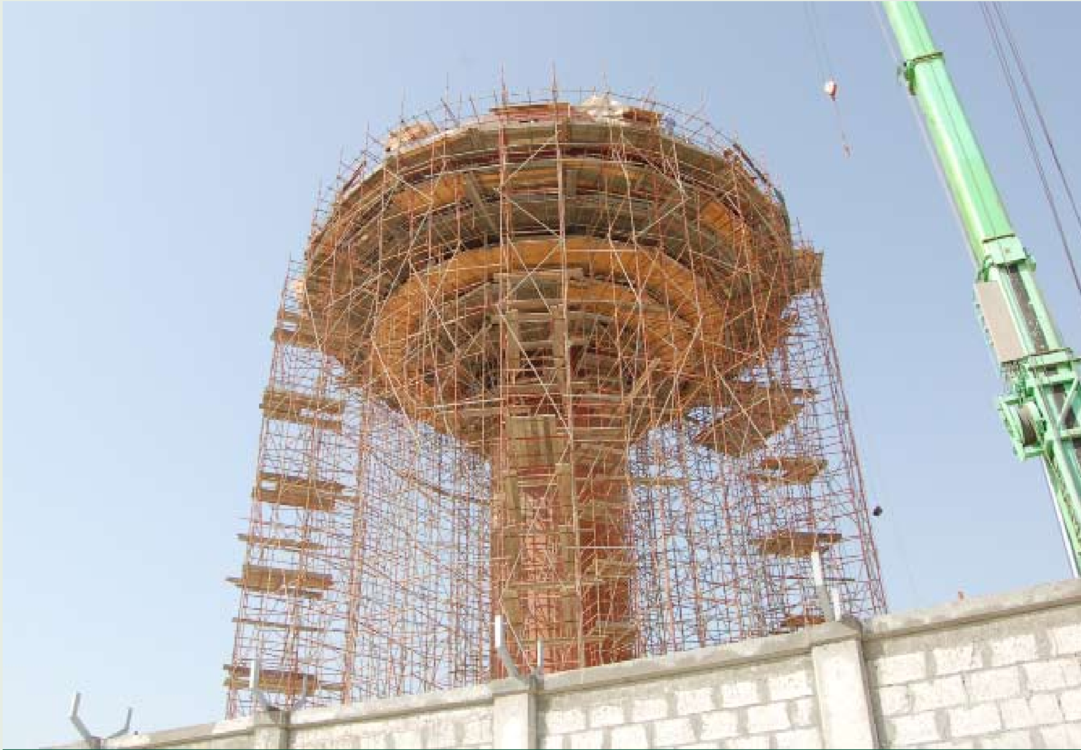
THE ELECTRICITY AND WATER AUTHORITY’S PORTABLE WATER NETWORK TANK CURRENTLY BEING INSTALLED AT THE ENTRANCE TO DURRAT AL BAHRAIN.
